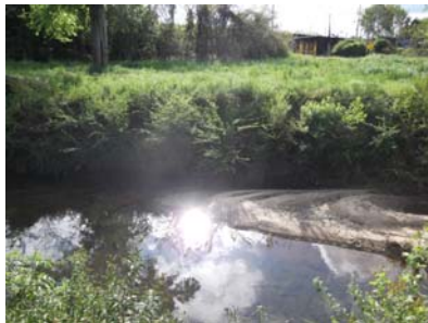
Sight 8, Bank 1: Bank slope greater than 45 degrees and 26%-50% ground cover. Is prone to erosion. B2
