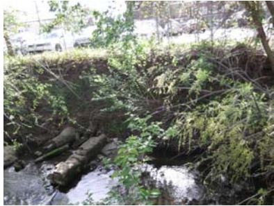
Sight 7, Bank 1: Bank slope greater than 45 degrees and 26%-50% ground cover. Is prone to erosion. B2
